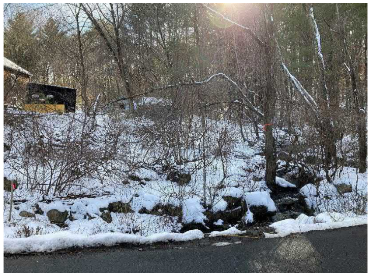
Photo 30 View southerly towards channel upgradient from culvert showing cobbles/boulders in vicinity of flagged BVW and steep winding channel through forest overstory. (1/17/23)
